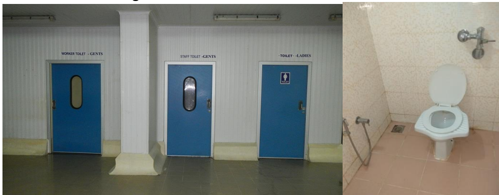
Figure 8: Gender specific toilets; clean toilet facility
