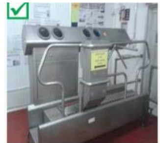
Figure 23: Automatic hand-washing and foot cleaning system
